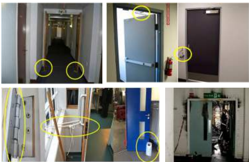
Photos depict actual rated door deficiencies discovered in healthcare facilities.
