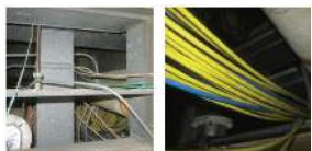
Two examples of fire dampers with wires running through them. This is a clear violation of NFPA 70 and NFPA 72.
