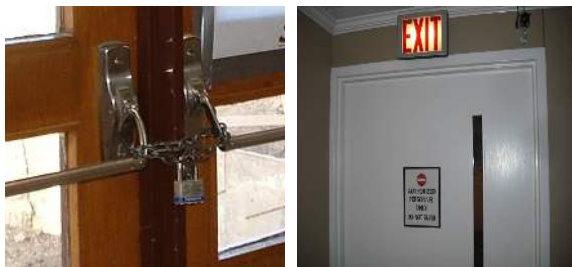
Photos depict actual deficiency examples discovered in healthcare facilities. The locked door is a life safety deficiency showing an immediate jeopardy to life .
