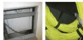
Two examples of fire dampers that are blocked and are no longer functional.
